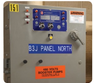
Control Panel & Electrical Panel Labels
